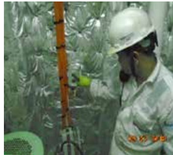
EMERGENCY FIRE PUMP WAS STARTED
